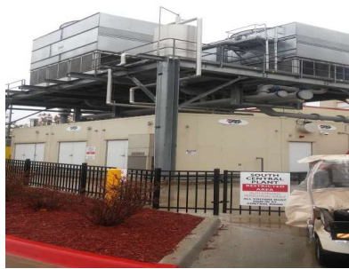
HR South Plant
